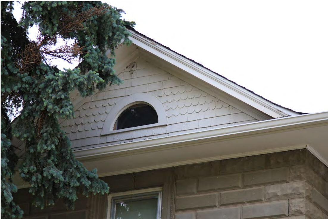
Front façade two-storey bay with rectangular and fish-scale wooden shingles and half-moon fixed wooden-sash window in front-gable peak. Also shown quoining with rough moulded concrete block, 2014 (DLA)
