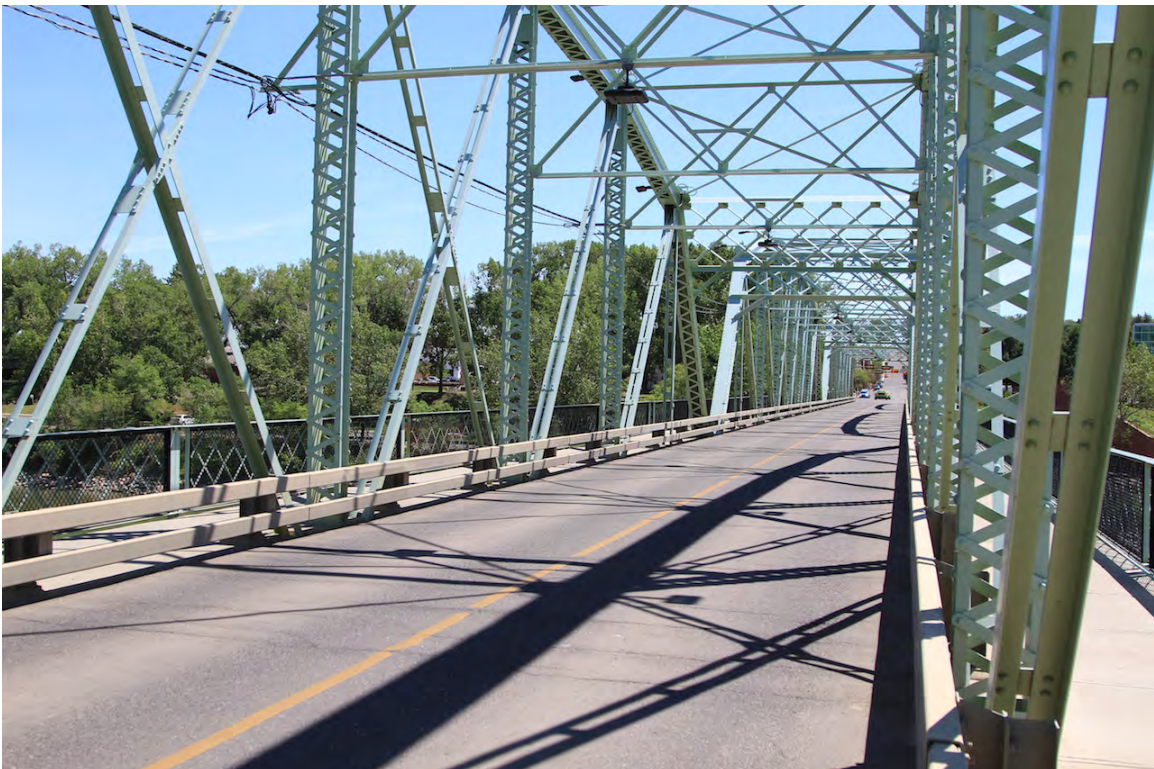
Two lane traffic deck with pedestrian walkways on the outside of the superstructure, June 2015 (DLA)
