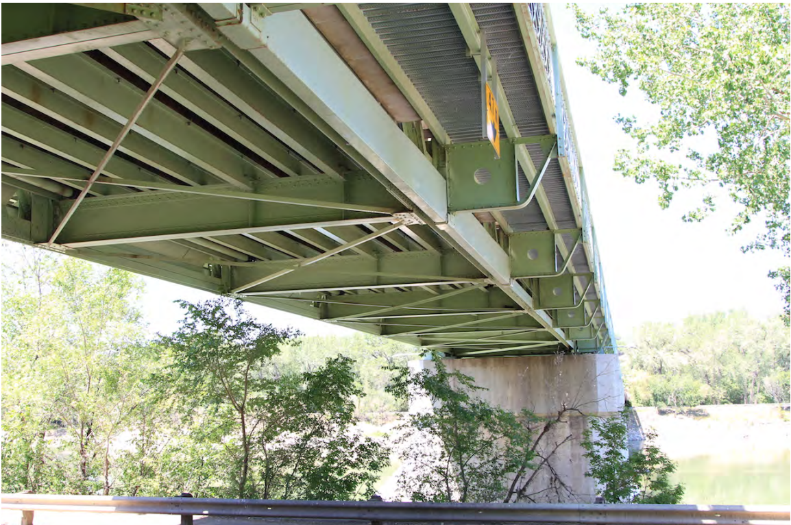
Underside of bridge deck showing bracing for sidewalk and replaced metal deck, June 2015 (DLA)
