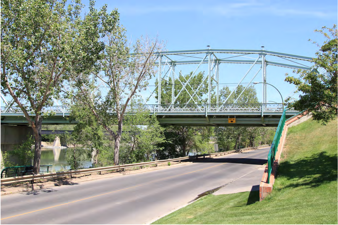
Southern end of bridge with River Road SE and pedestrian walkway running underneath, June 2015 (DLA)
