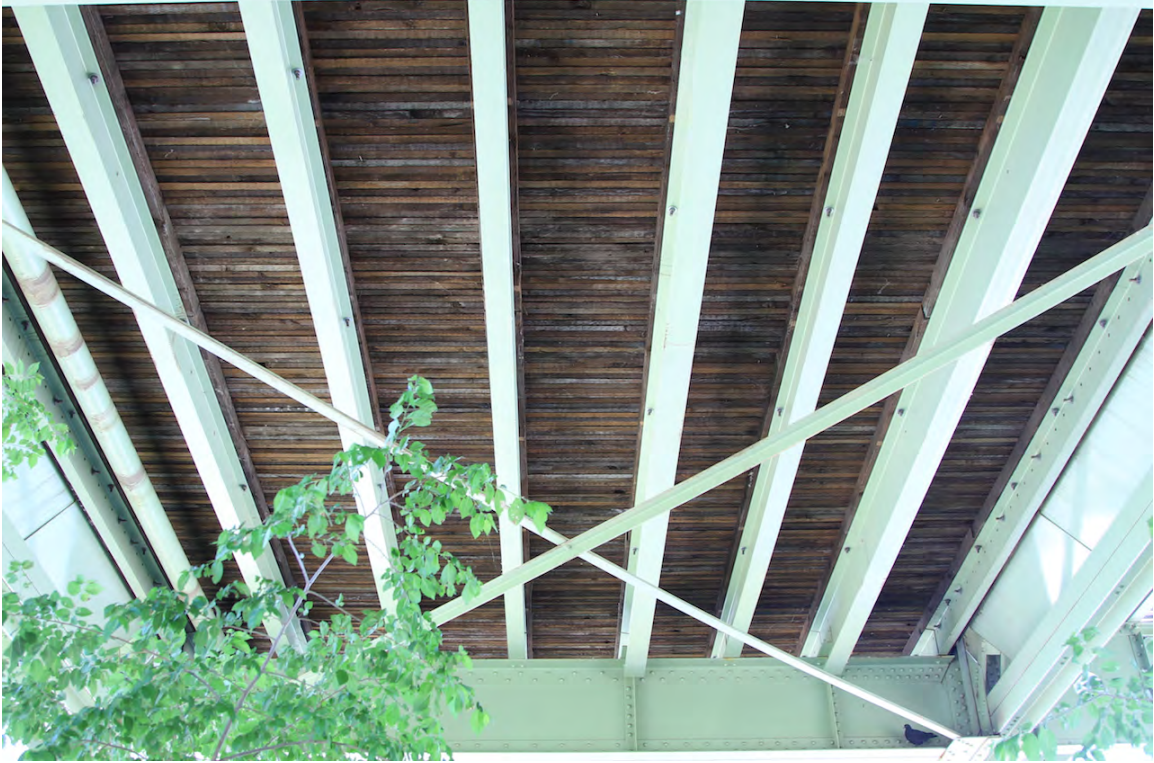
Underside of bridge deck showing wooden deck with steel stringers, June 2015 (DLA)
