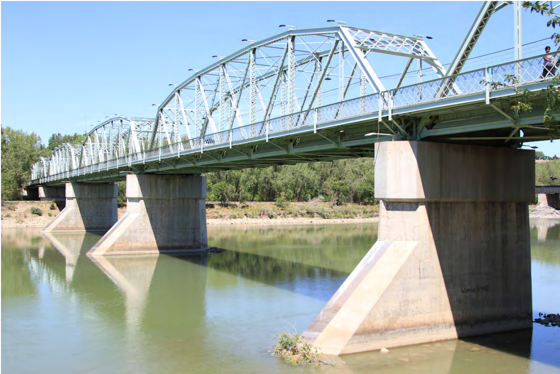
Finlay Bridge showing four of its five arched spans and concrete piers, June 2015 (DLA)
