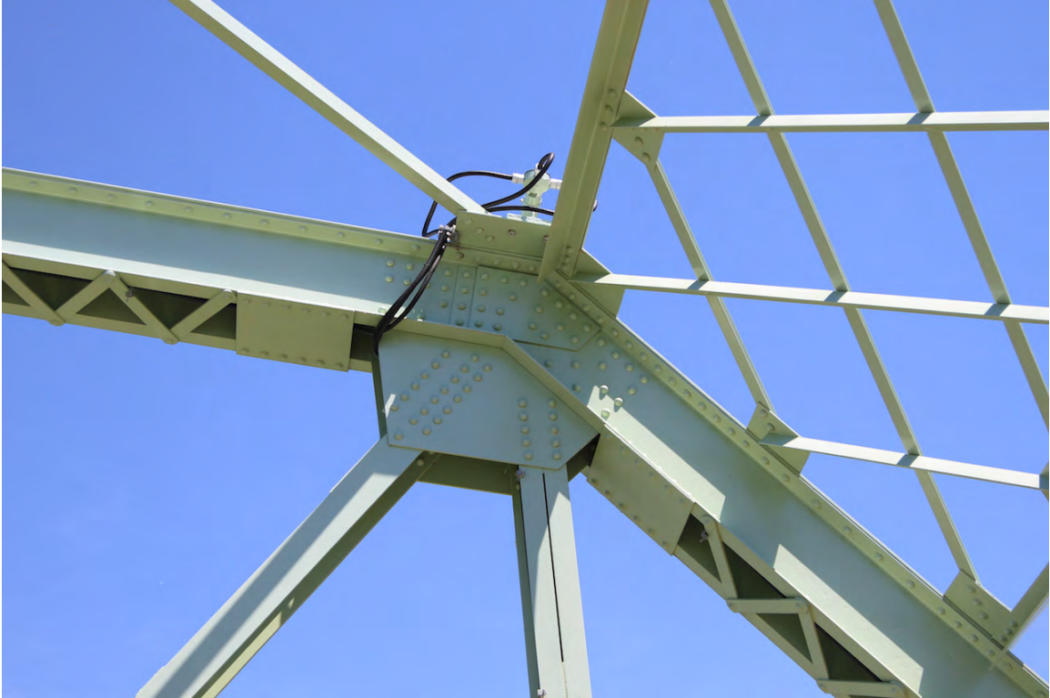
Example of riveting at connection of top chord, vertical members and diagonal and lateral bracing, June 2015 (DLA)
