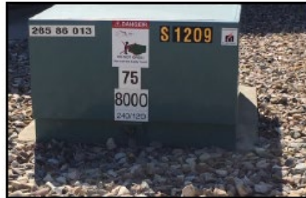
Single Phase Transformer
