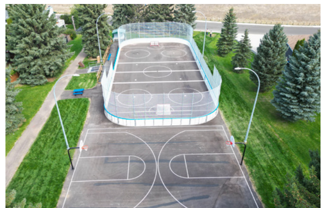
The rehabilitation of the multi-sport rink and court adds yet another distinction to Ross Glen Park, among the city's busiest activity destinations.
