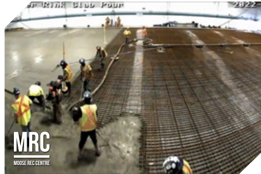
A deteriorated slab at the Moose Recreation Centre required a fresh pour prior to re-opening in September of 2022
