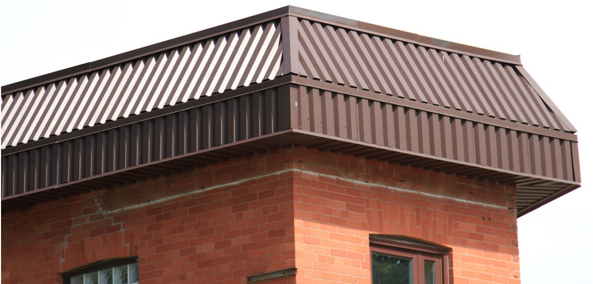
Corrugated metal cladding over brick parapet. Ghost outline of original cornice evident and past repointing of stepped crack at above window apparent, 2014 (Donald Luxton & Associates)
