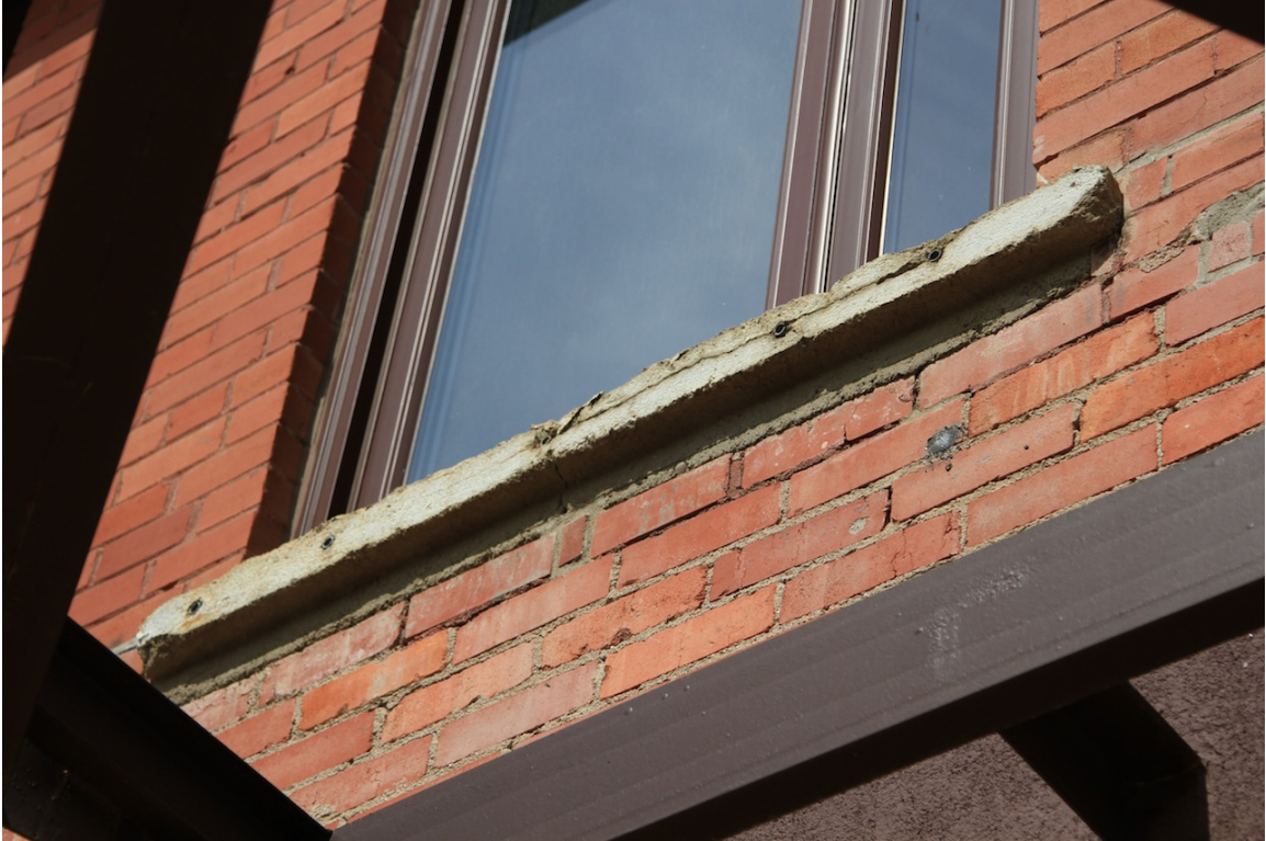
Deteriorated mortar and concrete sill below second storey window, 2014 (Donald Luxton & Associates)
