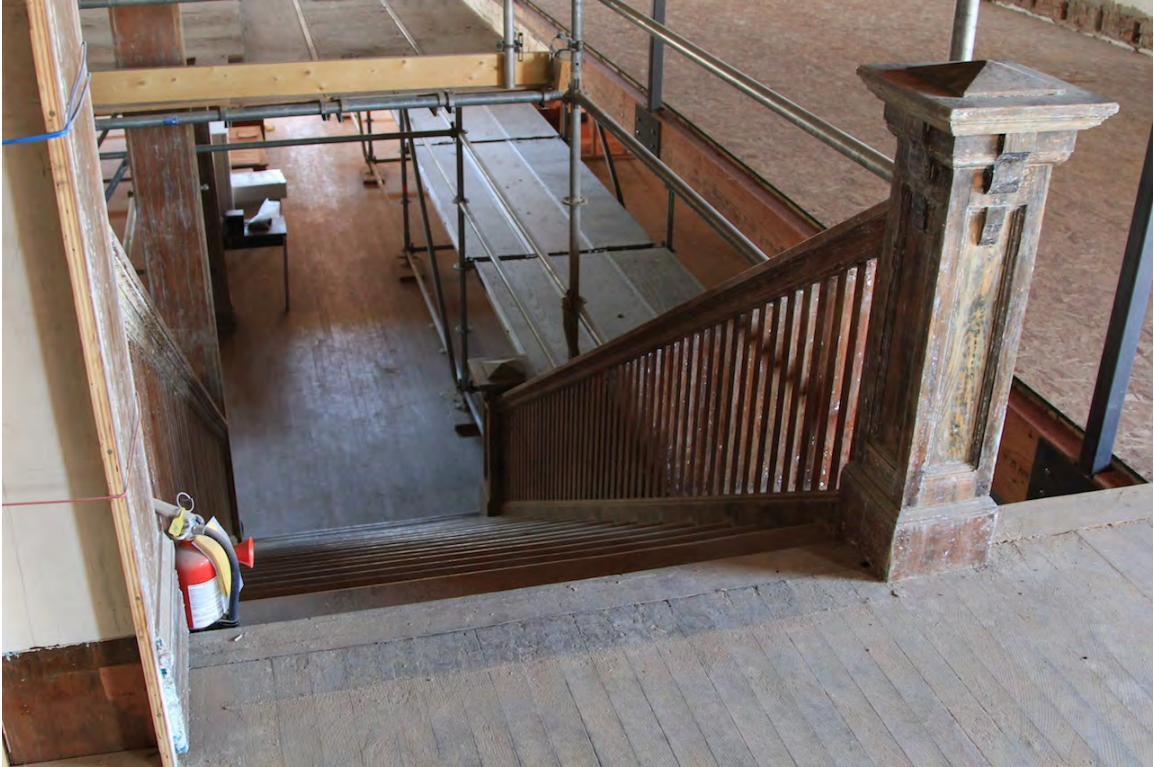
Wooden newel post of central stair on mezzanine level and square wooden spindle balustrade, 2014 (DLA)
