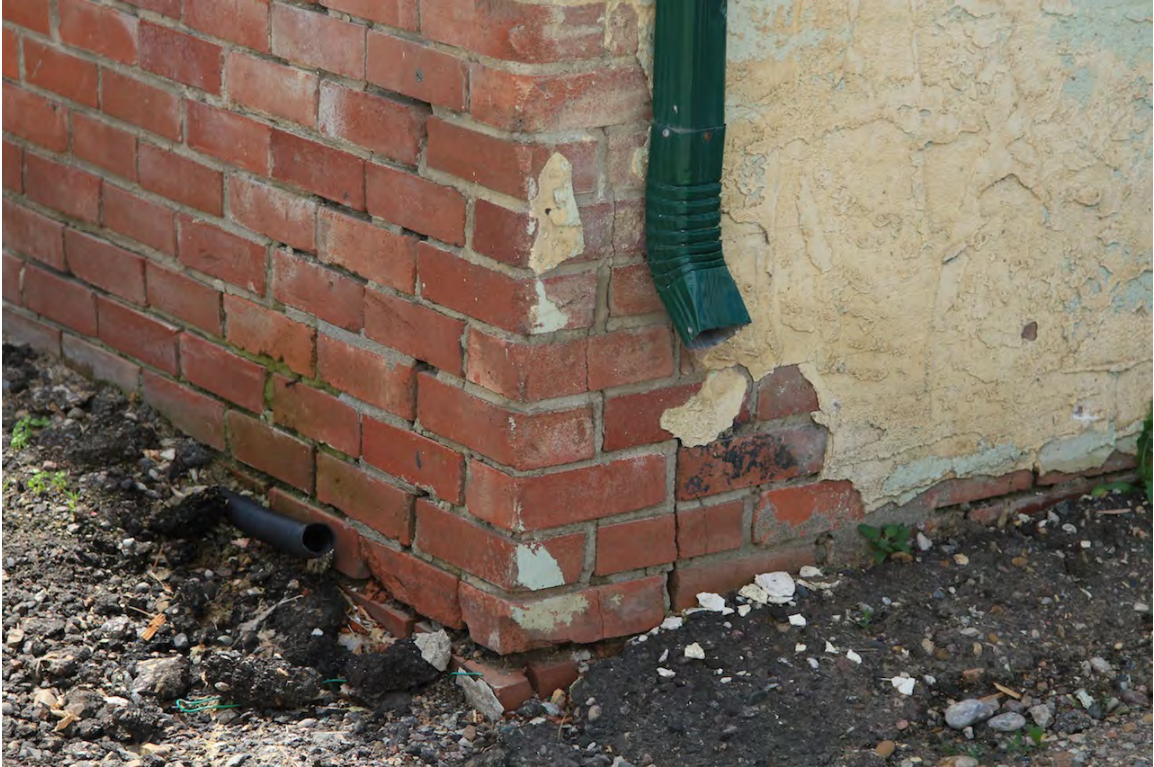
Poorly installed and maintained rwl at northeast corner of building, 2014 (DLA)
