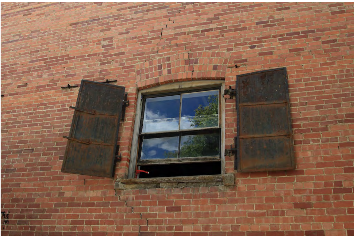
Segmental arch 2-over-2 single-hung wooden-sash window with metal shutters on east façade, 2014 (DLA)
